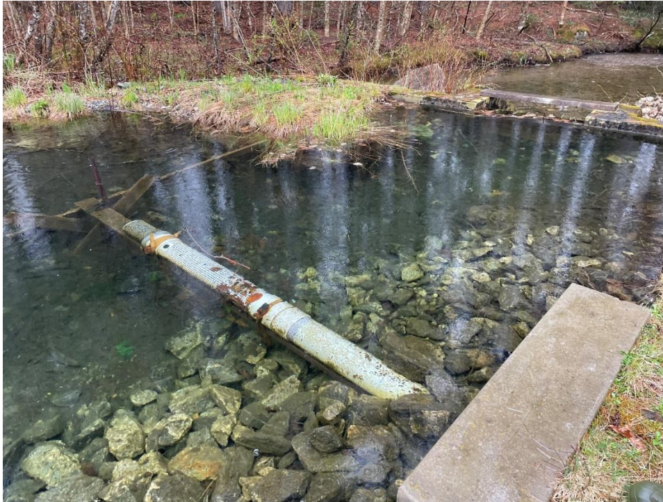
Figure 4-7: Cylindrical intake screen in Spring Reservoir
