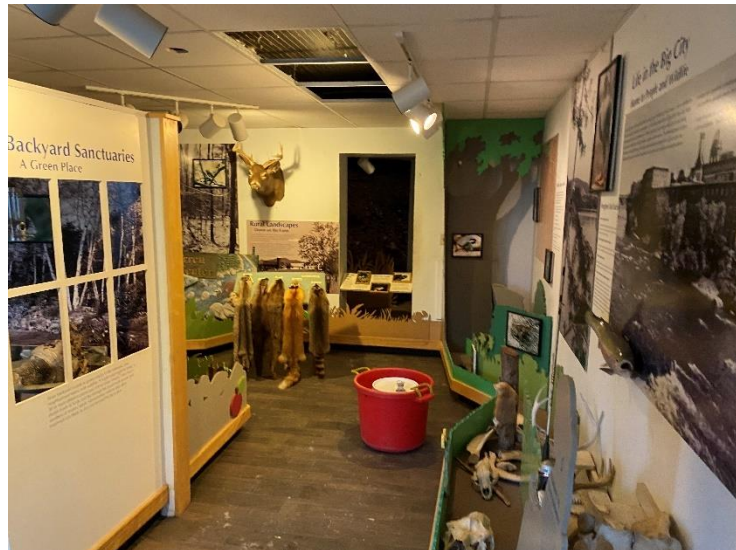
Figure 6-25: Visitor Center Missing Ceiling Tiles
