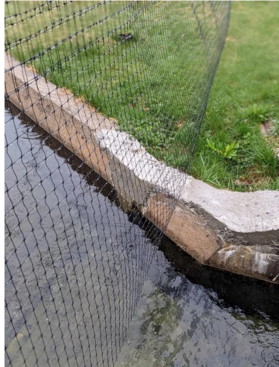
Figure 5-31: Previously Repaired Wall at Inlet to Middle Reservoir Pond
