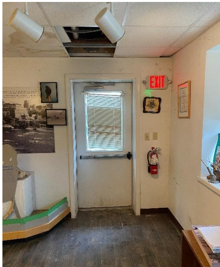
Figure 6-24: Visitor Center Water Damaged Ceiling Tiles
