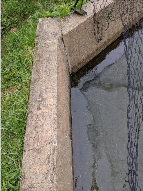
Figure 5-30: Typical Pond Wall Cracking at Angles/Corners
