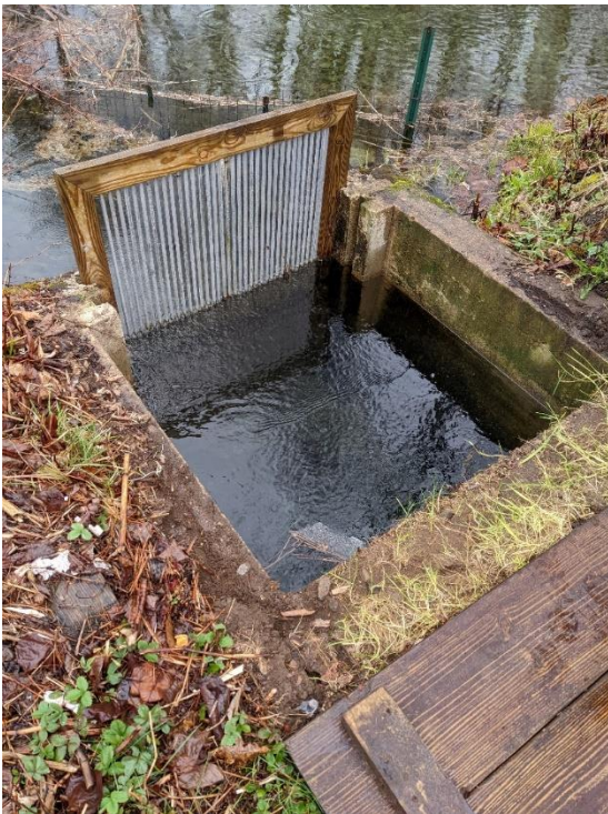
Figure 4-10: Screen Box in Pump 3 Reservoir
