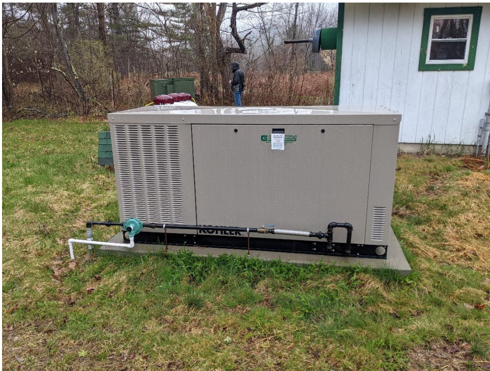
Figure 4-4: New 25kW Standby Propane Generator
