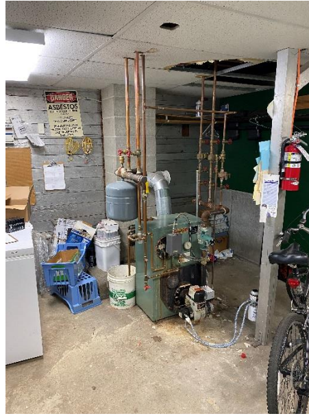
Figure 6-27: Mechanical Room missing and broken ceiling tiles
