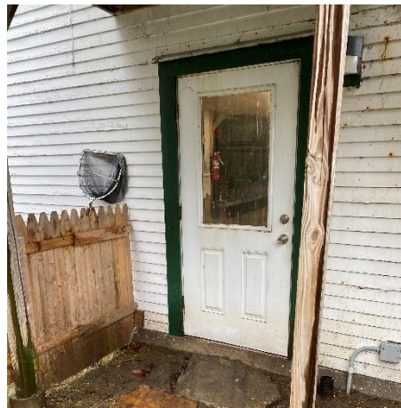
Figure 6-23: Rusted Hinges on Door to Mechanical Room
