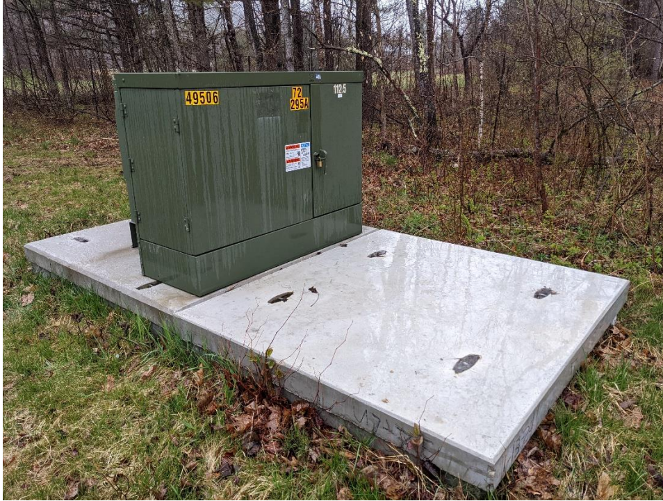
Figure 4-3: Transformer and Foundation at Well/Pump House #2
