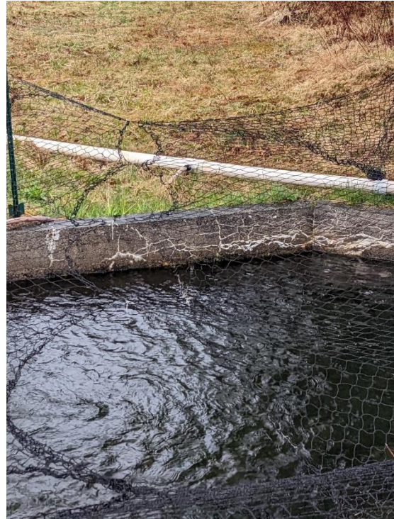
Figure 5-34: Concrete Deterioration at Block 2 Ponds
