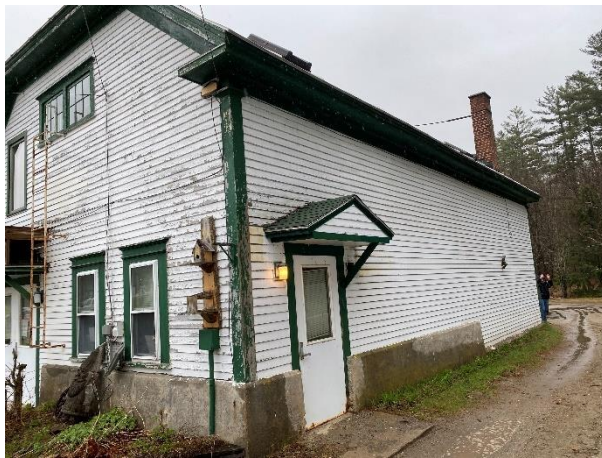
Figure 6-22: Rusty bottom of door to Visitor Center
