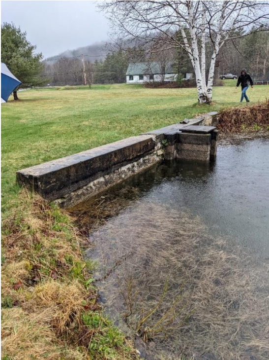
Figure 5-36: Impoundment/Outlet Box at PR Pond
