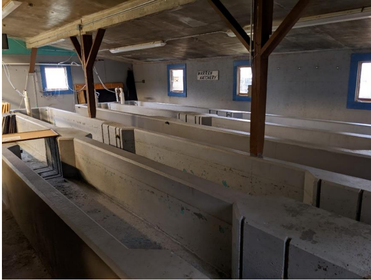
Figure 5-11: Hatch House Interior Raceways in Addition at Back
