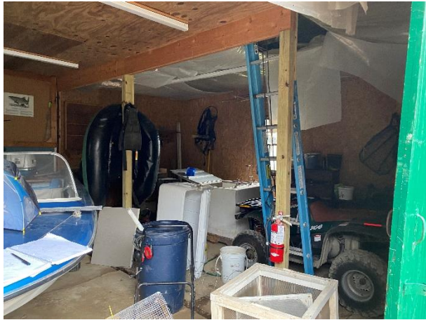
Figure 6-2: Cracked Floor and Plastic Sheetting
