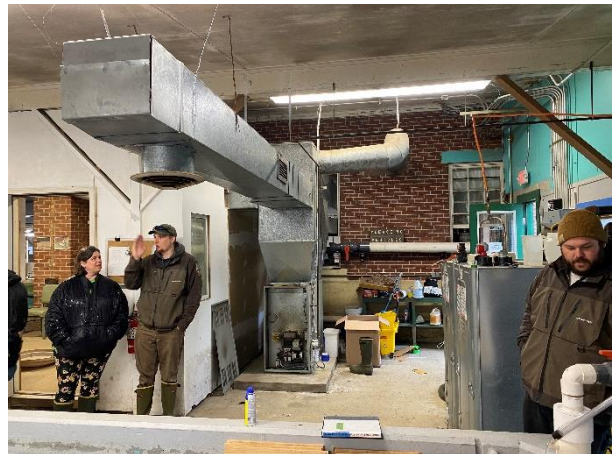
Figure 5-27: Rear Tank Room Mechanical / Electrical Space
