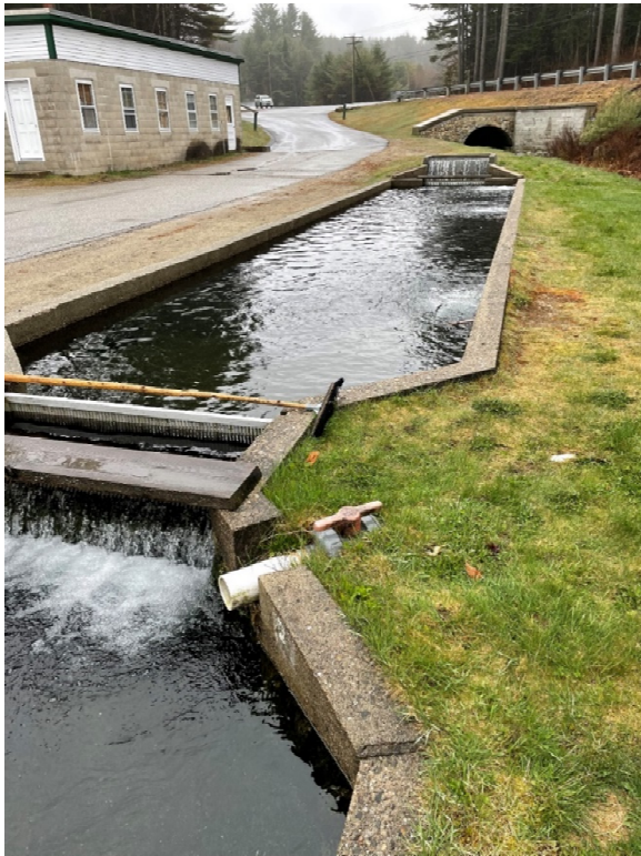
Figure 5-11: Raceway B-2 Supply Valve
