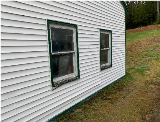
Figure 7-7: Visitor's Center Garages Damaged Windows
