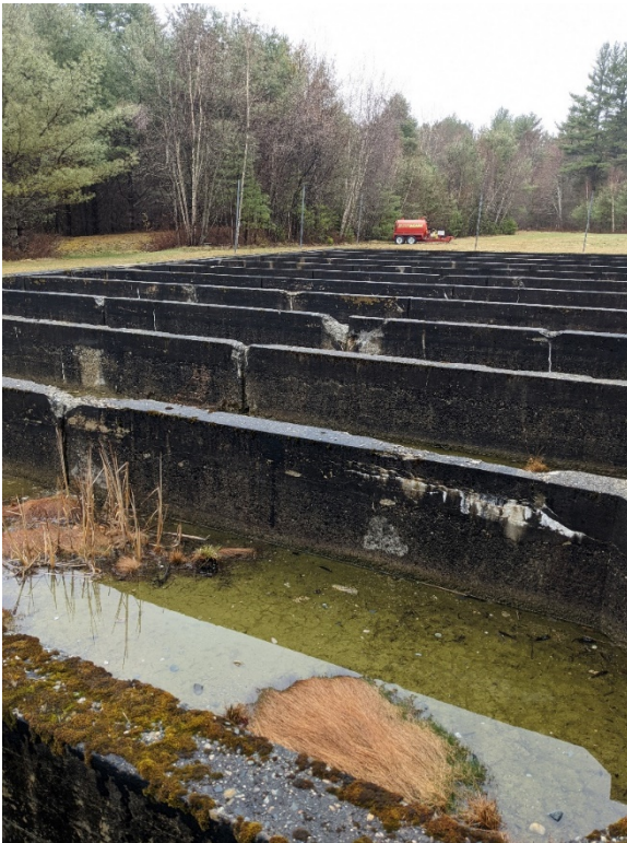
Figure 5-9: Abandoned A-Series Raceways
