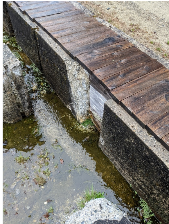
Figure 5-10: Covered Bypass Channel at A-Series Raceways
