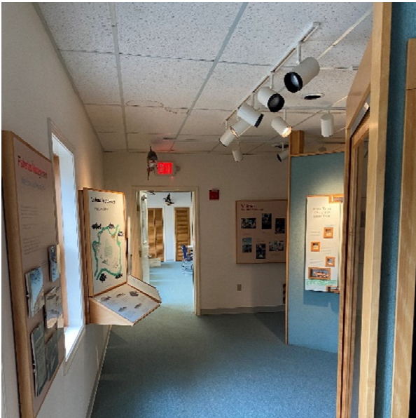
Figure 3-4: Display Room with water damaged ceiling tiles
