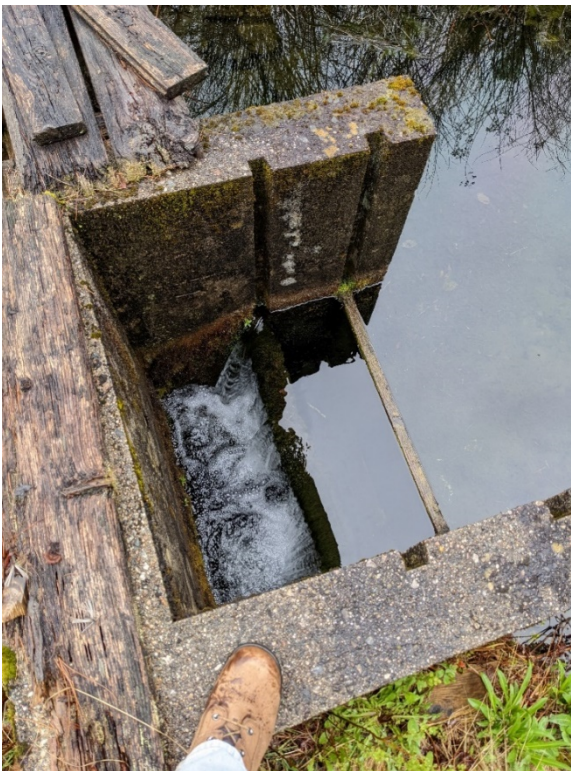
Figure 4-3: Concrete Headbox of Covered Spring
