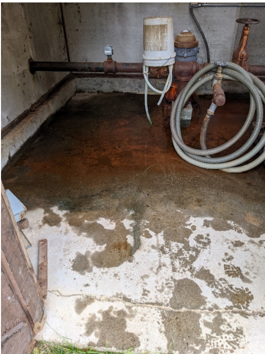
Figure 4-9: Interior of Well/Pump House
