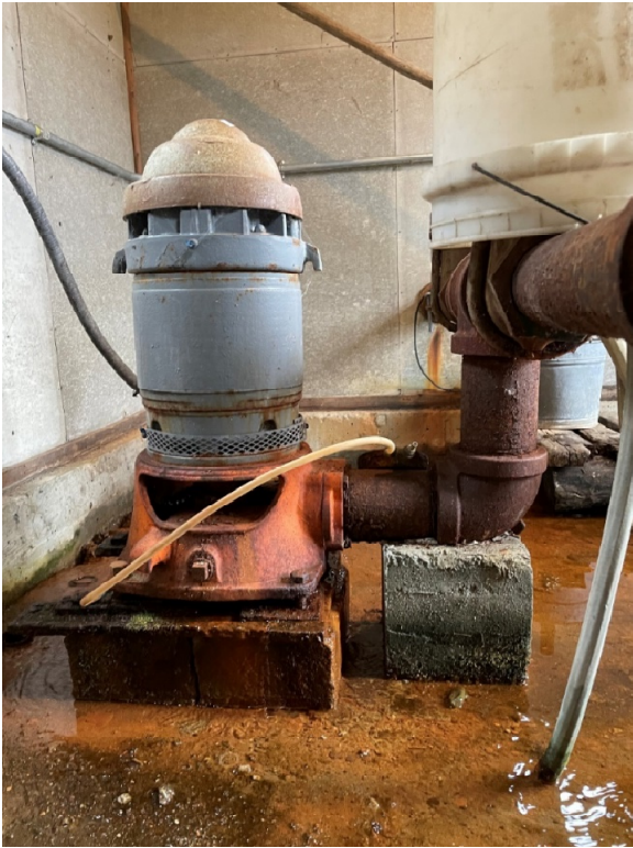
Figure 4-7: Production Well Pump Discharge Head
