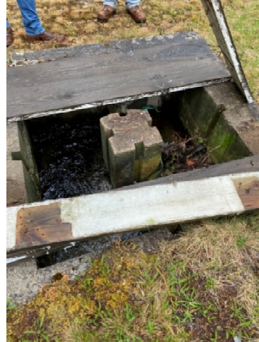
Figure 4-11 Right Spring Junction Box
