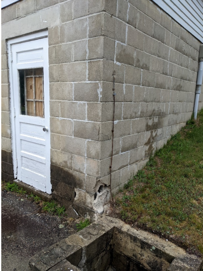
Figure 5-6: Cracking of Masonry Block at Hatchery SW Corner
