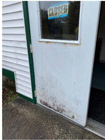
Figure 3-5: Rusted door at Exit Vestibule
