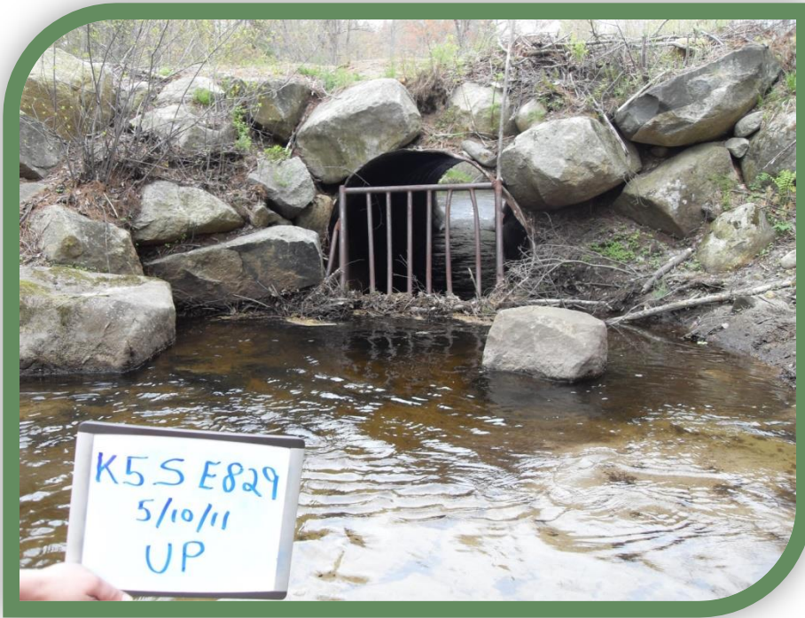
Undersized and screened culvert inlet, Falls Brook, Swanzey on May 10, 2011.
