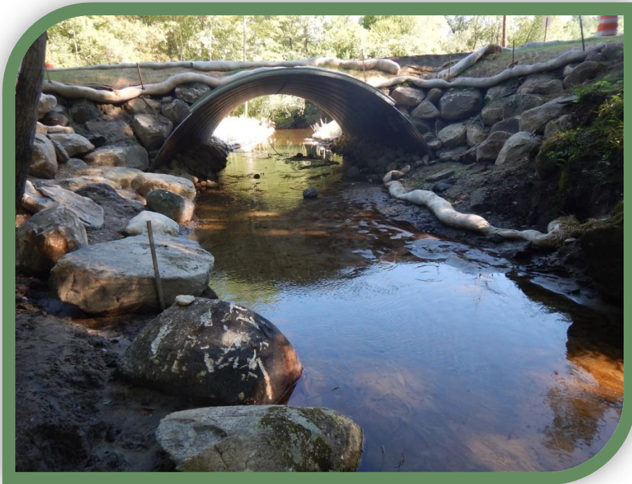
Culvert replacement with a 23' open bottom arch culvert under Hale Hill Road, Falls Brook, Swanzey
