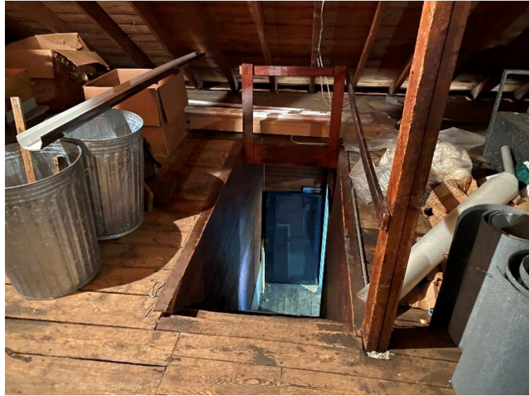
Figure 5-23: Attic Stairs with missing railing and no handrails
