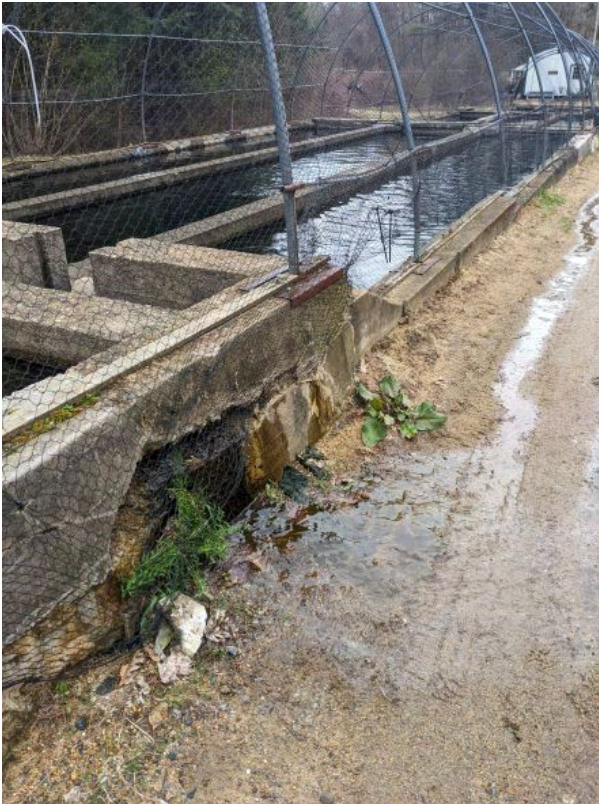
Figure 5-39: Severe leaking from north outside wall at B-Series
