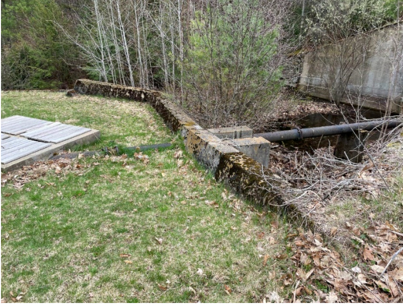
Figure 4-4: Minor Spring Concrete Distribution Box/Inlet Piping Below Crossing of RT 132
