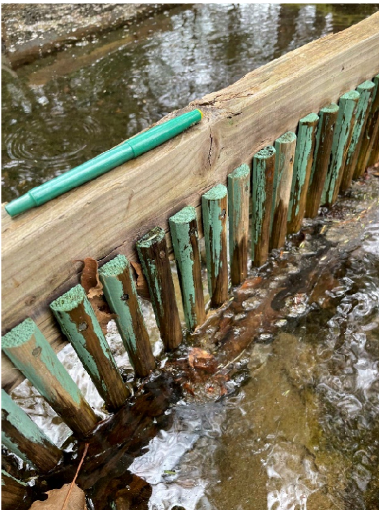
Figure 4-8: Wooden Stoplogs at Screen Upstream of Wood Framed Inlet at Minor Spring
