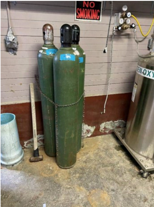
Figure 5-4: High Pressure Oxygen Cylinders
