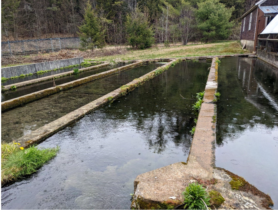
Figure 5-32: Unprotected “outside” raceways in Raceways A-3, used for treatment/settling
