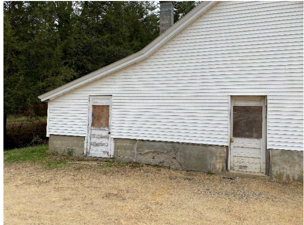
Figure 5-7: North Facade Foundation Cracks and Spalling
