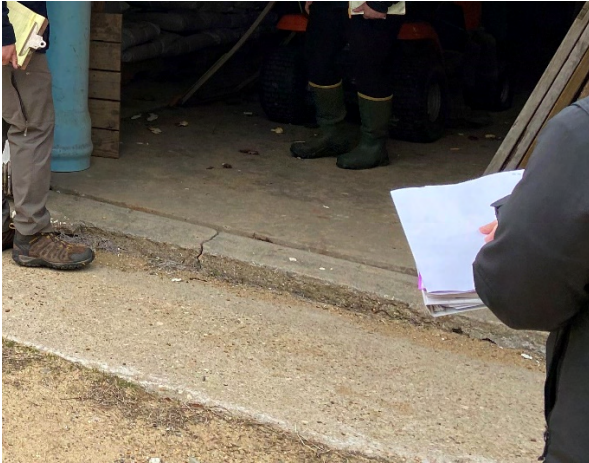
Figure 7-2: Example of cracking at foundation curb
