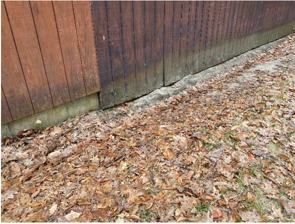
Figure 7-11: Damaged Wood Paneling Base
