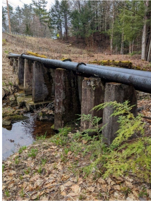
Figure 4-11: B-Series inlet piping shifted at support cradles at upper creek crossing
