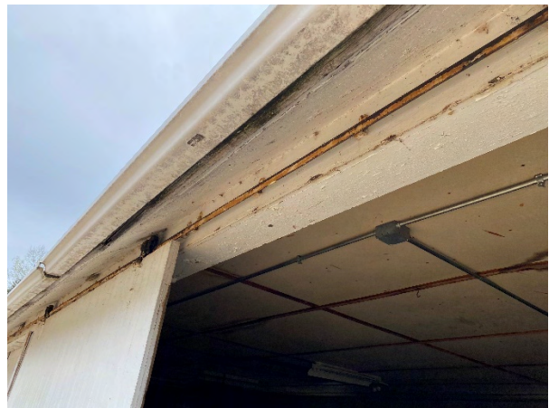
Figure 7-5: Rusted door slide rail and damaged gutter
