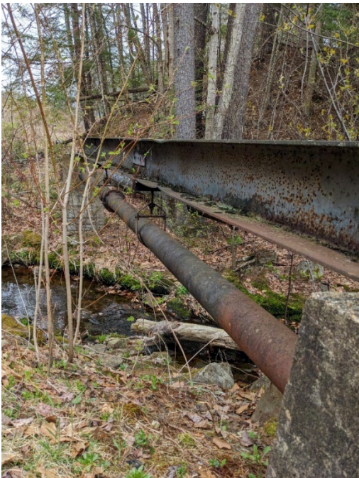
Figure 4-12: B-Series inlet piping at lower creek crossing
