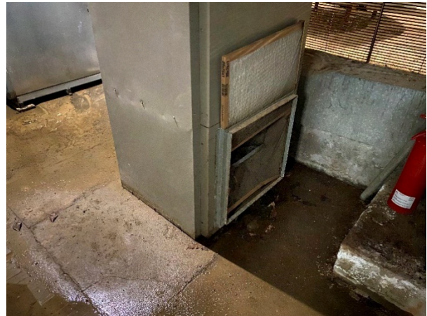
Figure 5-19: Mechanical Room Floor & Screens
