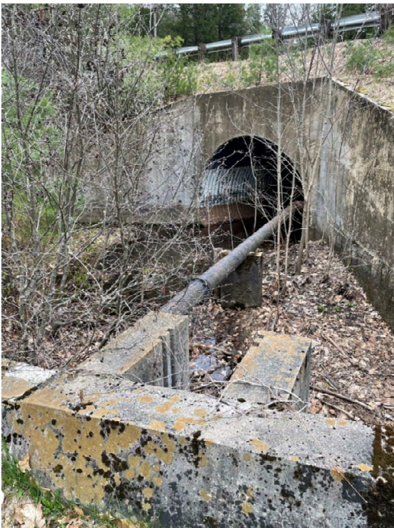
Figure 4-5: Pipe Support Across RT 132 from Minor Springs
