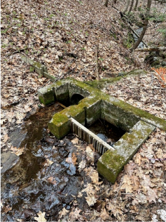
Figure 4-1: Major Springs' Typical Stoplog Structure
