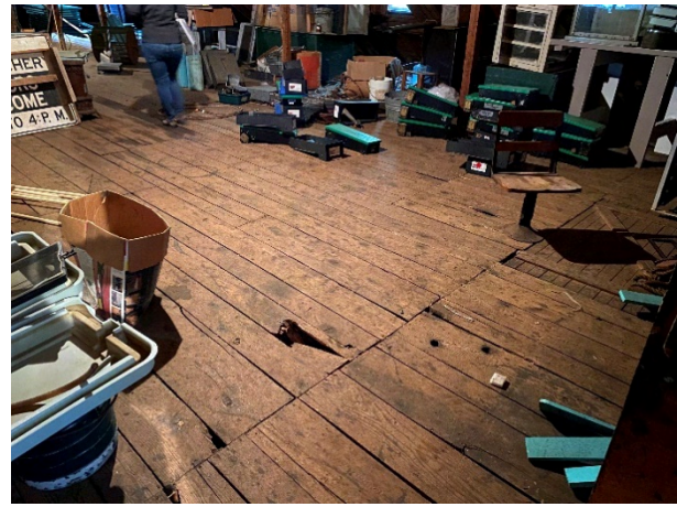
Figure 5-25: Attic broken floor boards
