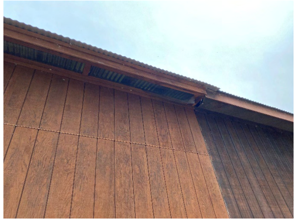
Figure 7-12: Damaged Soffit Screening
