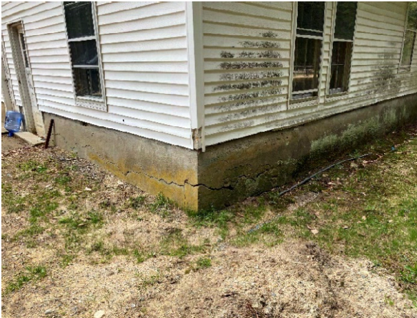
Figure 5-6: SE Corner Foundation Cracks Hatch House Main Production Rearing Area
