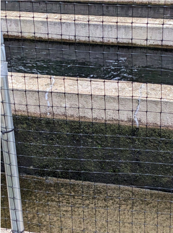
Figure 5-44: Previously repaired concrete surfaces at C-Series upper raceways
