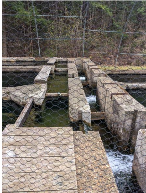
Figure 5-40: Concrete spalls, cracking and deterioration at B-Series baffles
