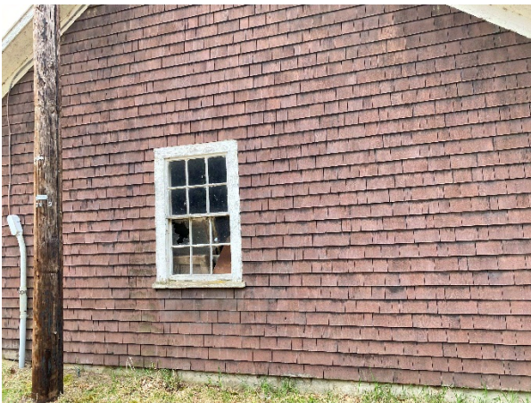
Figure 7-4: Broken windowpanes at east elevation
