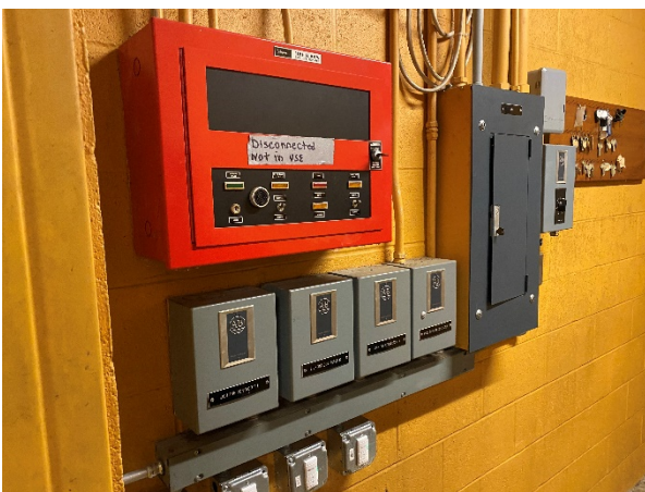
Figure 5-23: Electrical Room North Wall with Disconnected Fire Alarm Panel
