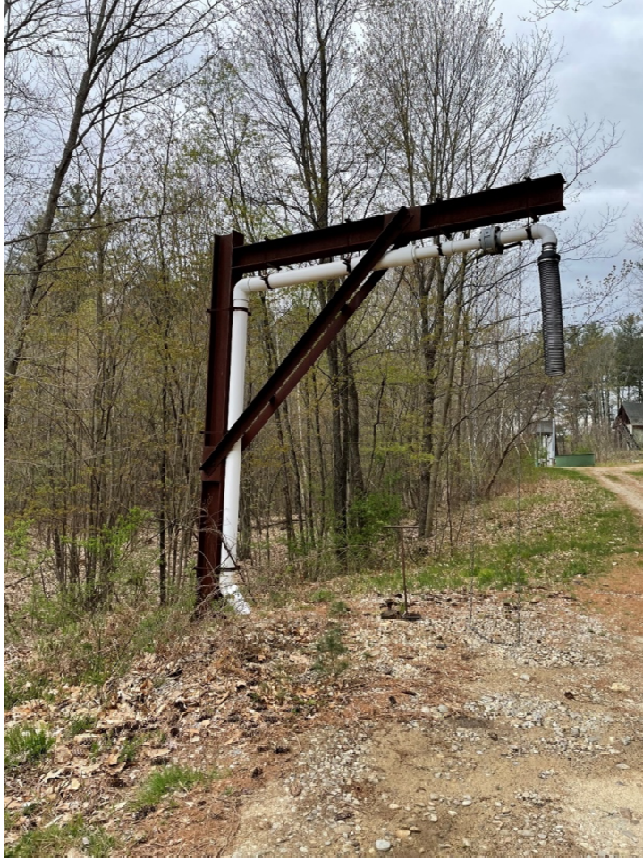
Figure 4-9: Truck Fill with Slow Exposed Leak
