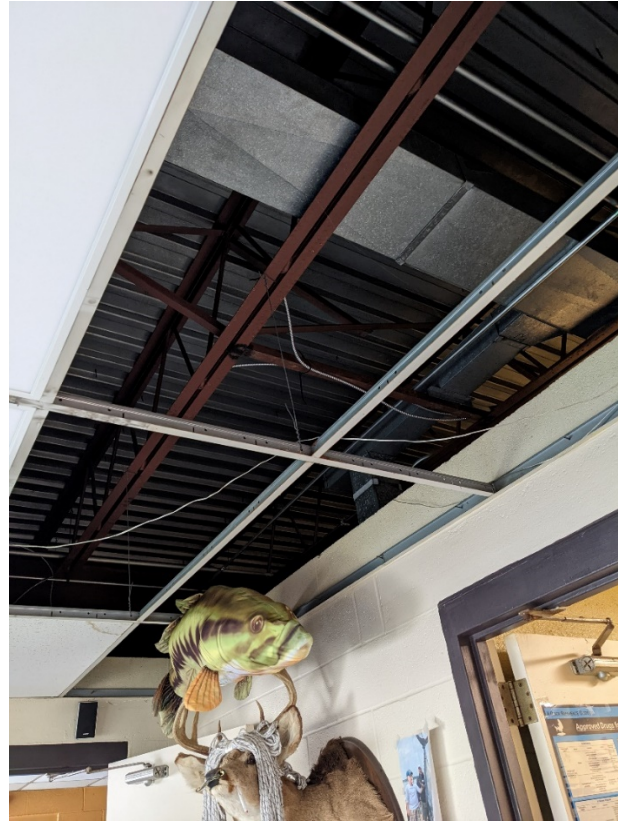
Figure 5-6: Area of Roof Leak in Lounge Area, with Removal of Suspended Ceiling
