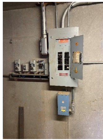
Figure 5-22: Electrical Panel in Addition
