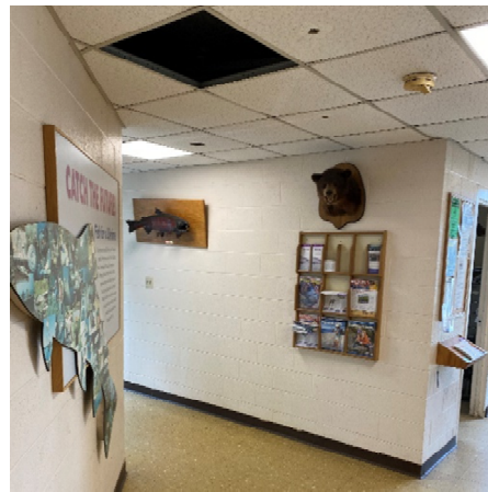
Figure 5-11: Missing Ceiling Tiles and Holes in Public Areas
