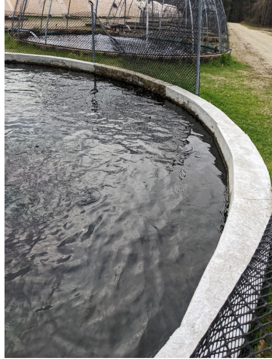
Figure 5-31: Previous Concrete Repair at Lower Area Tank Walls (Show Tank)
