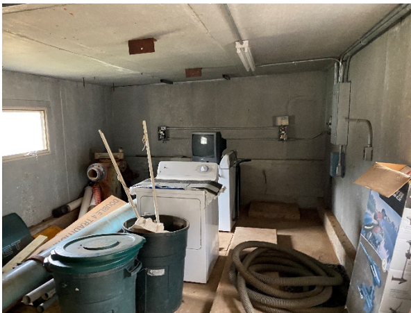
Figure 5-21: Electrical Panels in Addition
