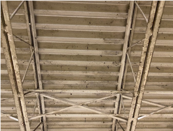
Figure 5-12: Black Mold Spots on ceiling in tank room
