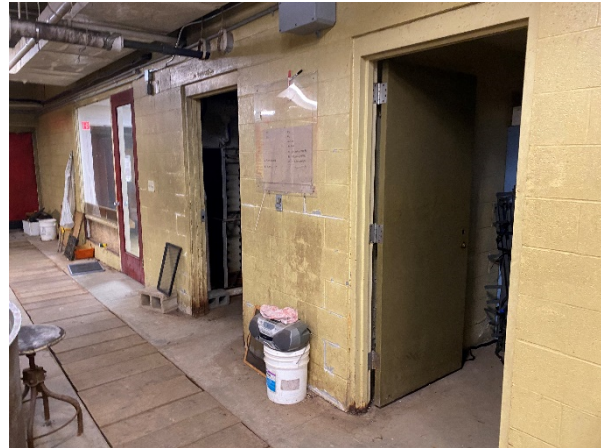
Figure 5-13: Black Mold Stains on walls in tank room
