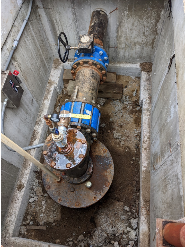
Figure 4-3: Field Well (No. 5) Inside Concrete Vault (in use)
