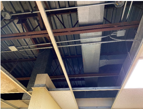
Figure 5-10: Missing Ceiling Tiles in Crew Area
