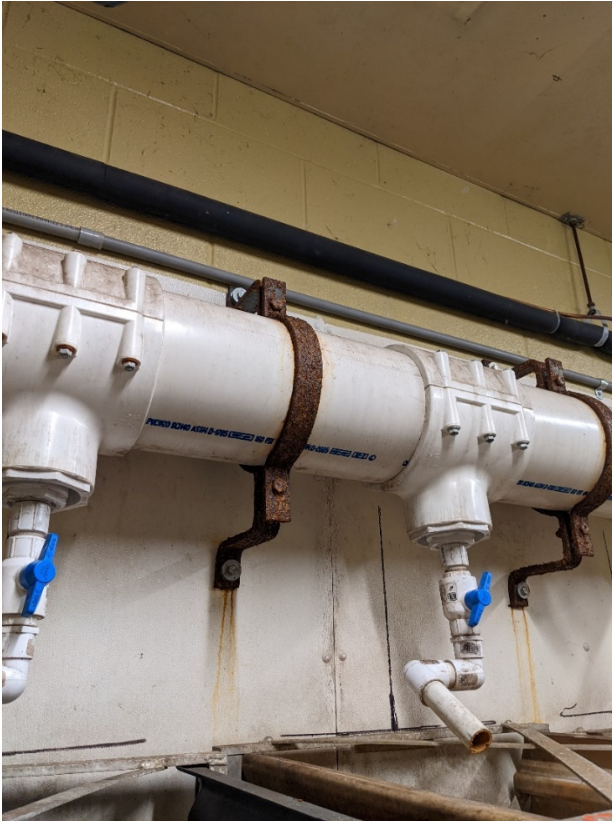
Figure 5-5: Rusting Hangers in Incubation Room
