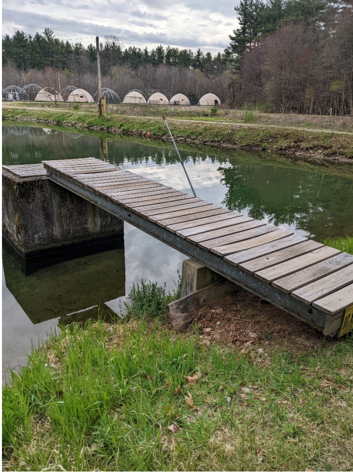
Figure 5-34: Access Walkway to West Pond Outlet Box; East Pond (treatment) in Background
