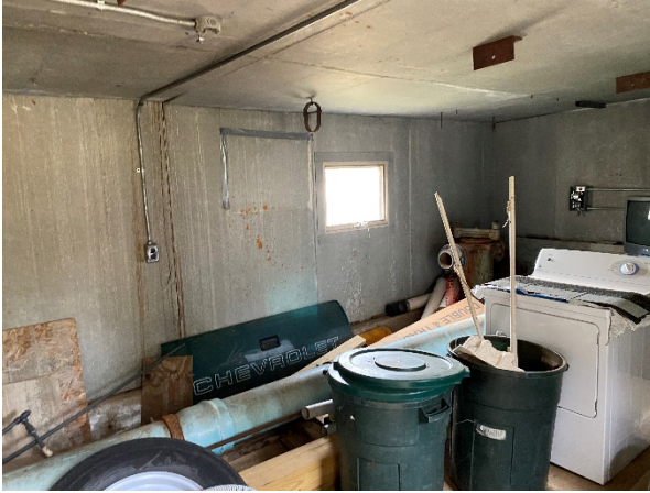
Figure 5-19: Interior of Addition showing water stains and rusted hangers
