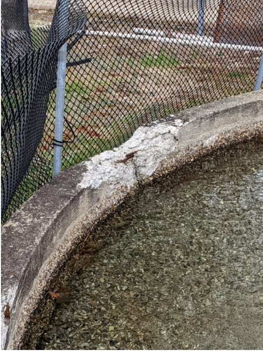
Figure 5-30: Typical Concrete Deterioration Upper Area
