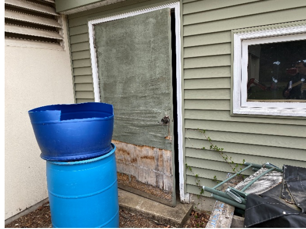
Figure 5-20: Rotted door to addition
