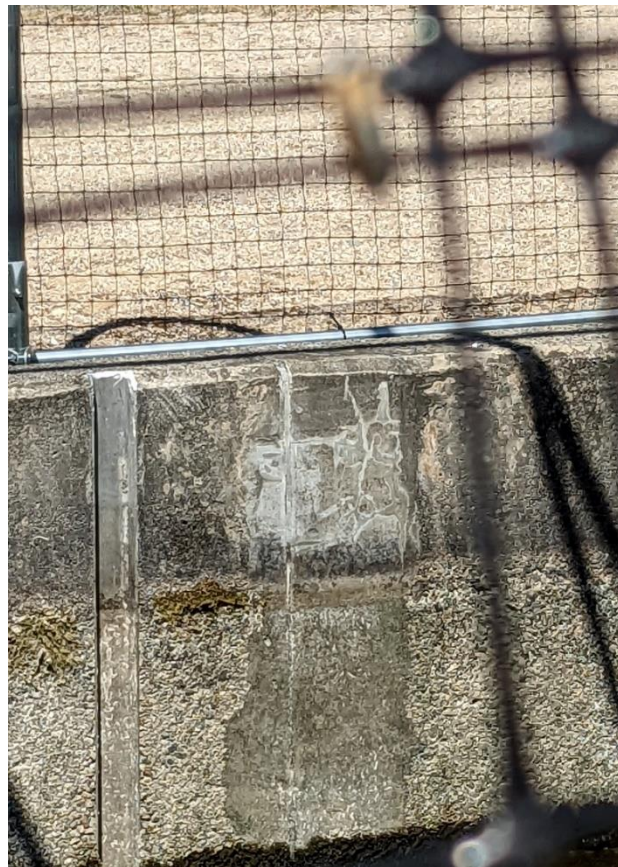
Figure 5-6: Young's Raceway Concrete Condition
