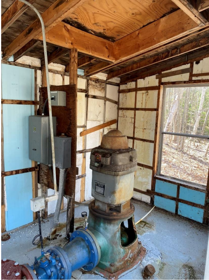
Figure 4-7: Well House #2 Interior
