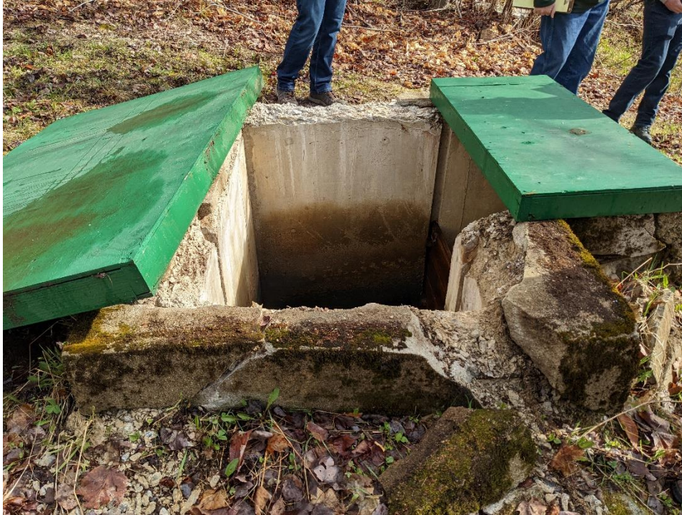
Figure 4-2: CB Distribution Box
