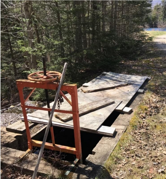
Figure 4-12: Gated Pipeline from Diversion Pond to Raceways
