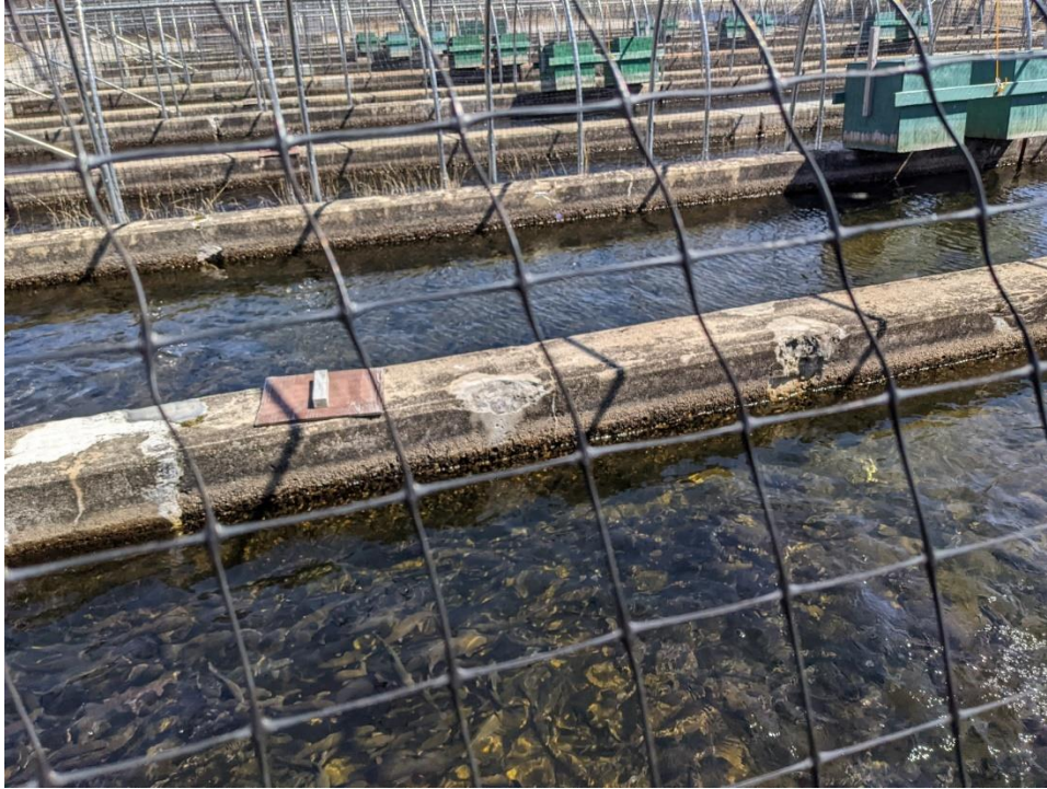
Figure 5-16: West Branch Raceways Concrete Condition
