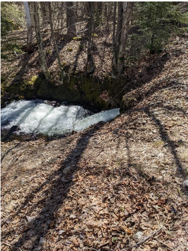
Figure 5-14: Outfall 005 Embankment at End of Canal C
