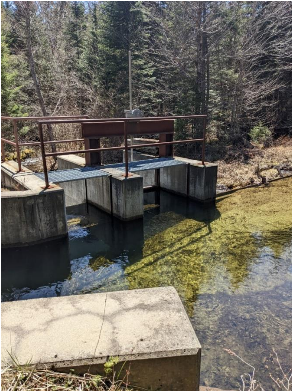
Figure 4-9: Double-Box Concrete Spillway (intake box is to the left of image (river left side))
